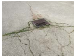
4) CB IN WEST PARKING LOT
