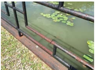
3) RUST ON RAILING
