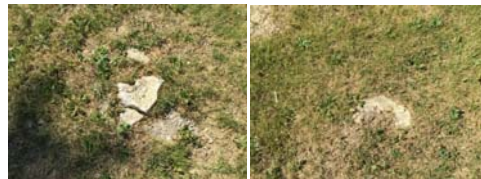
11) CONCRETE DEBRIS IN GRASS
