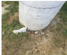
1) PARKING LOT LIGHTING
