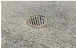
2) PARKING LOT CATCH BASIN
